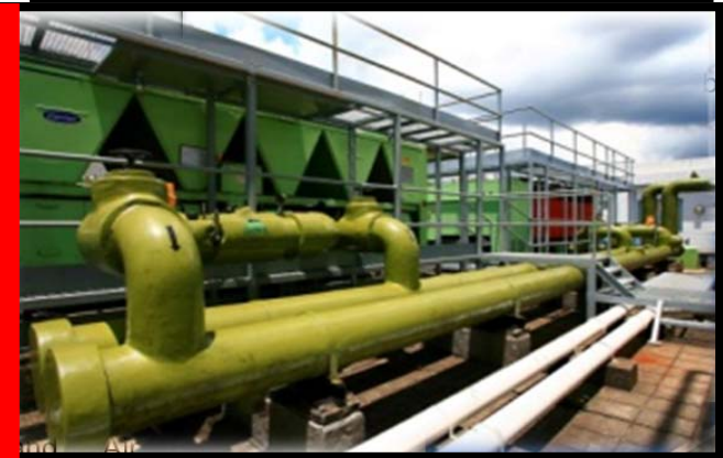
冷氣系統 (Air-Conditioning System)
